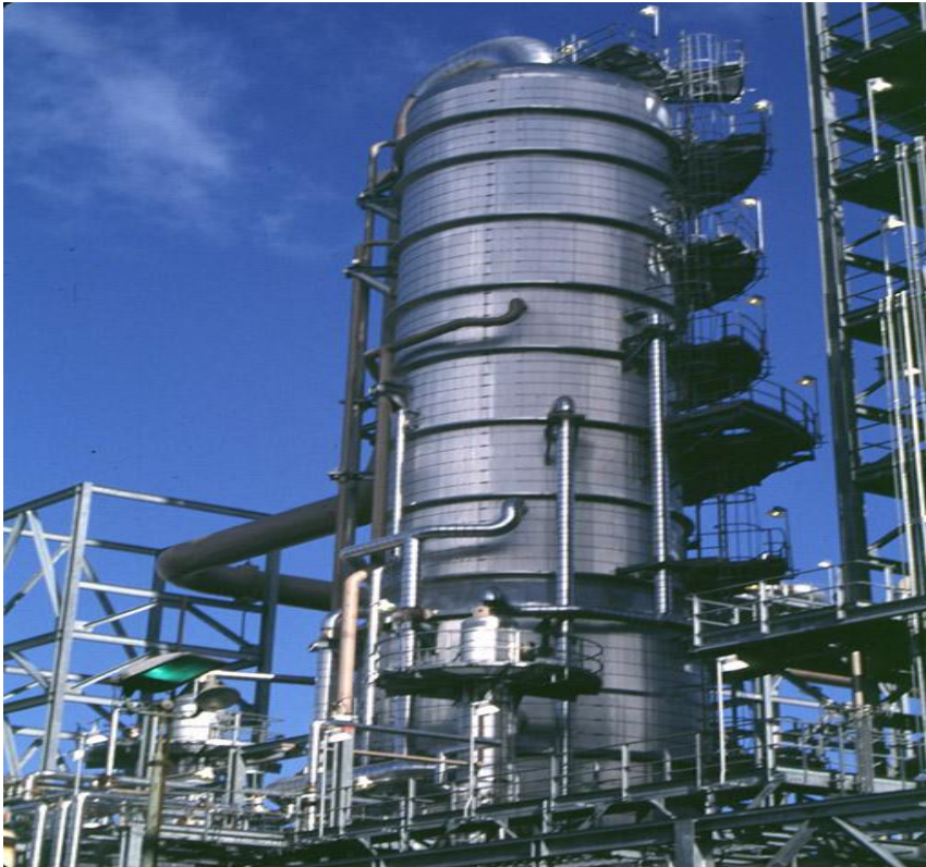
Fluid catalytic cracking distillation unit Source: Chevron (copyrighted)
